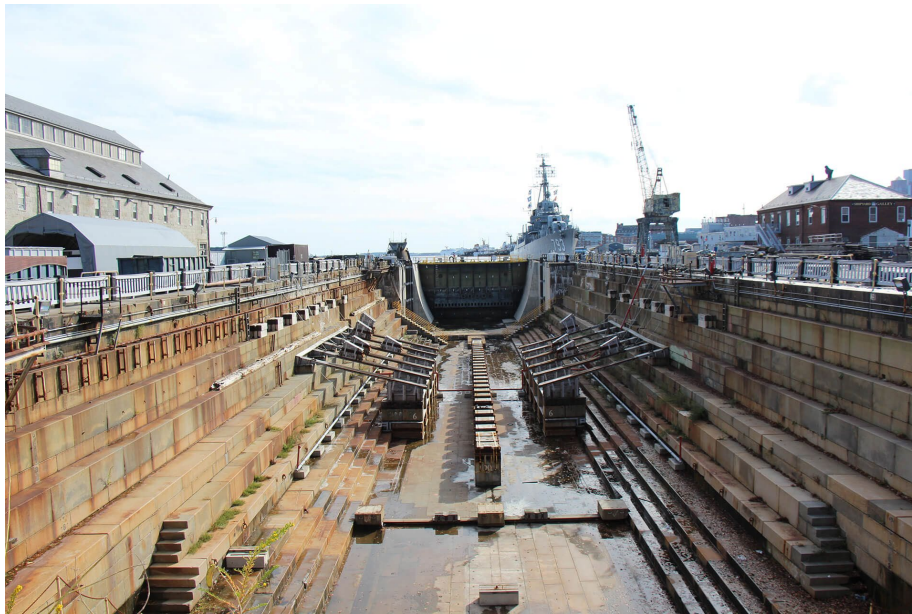
Figure 2.1.2 Graving Dry Dock Lined with Keel and Side Blocks, including the Dock Gate at the far end of the basin. Dry Dock #1, Charleston Shipyard, constructed in 1833.
