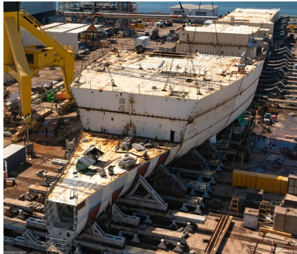
Figure 3.5.1: US Navy LPD Undergoing New Construction atop Railed Strongbacks, Ingalls Shipyard ( https://www.seaforces.org/usnships/lpd/LPD-30-USS-Harrisburg.htm )
